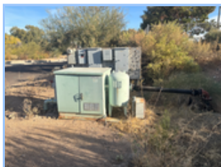
Pump cabinet and electrical gear
