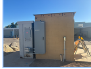
Exterior Lighting Controls
