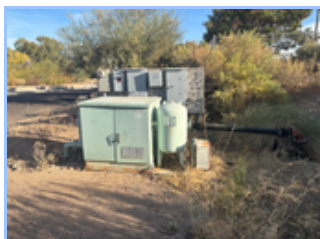
Pump cabinet and electrical gear
