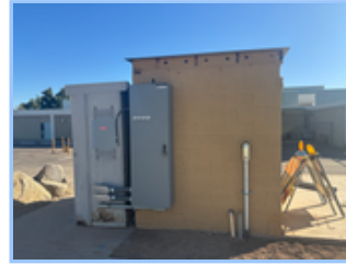
Exterior Lighting Controls
