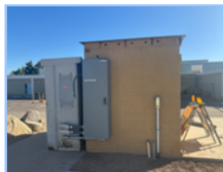
Exterior Lighting Controls
