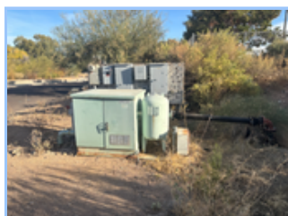
Pump cabinet and electrical gear
