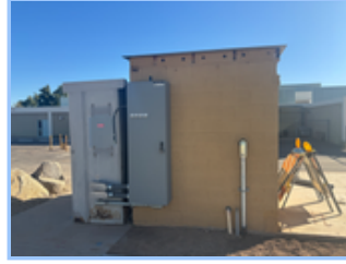
Exterior Lighting Controls
