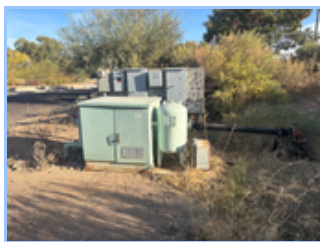
Pump cabinet and electrical gear
